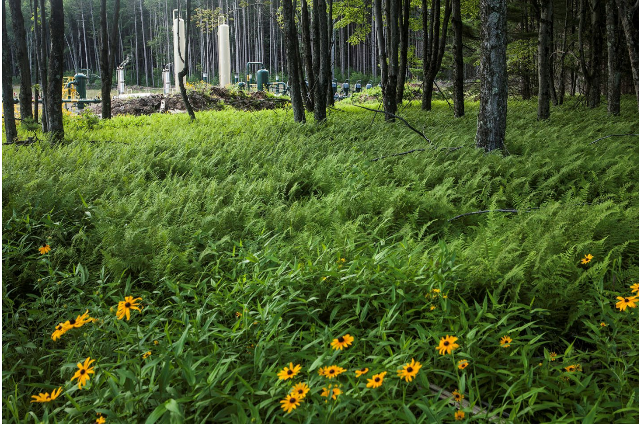
Figure 3. Separators and other gas-processing components on a well pad inside Tiadaughton State Forest, Lycoming County, Pennsylvania. July 17, 2014.
